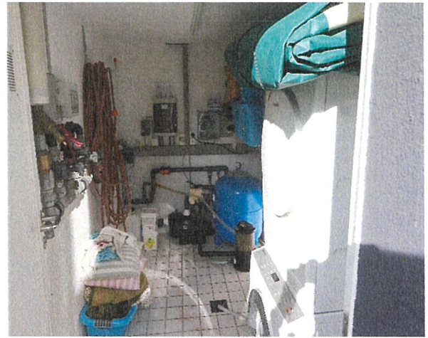
LOCAL TECHNIQUE PISCINE
